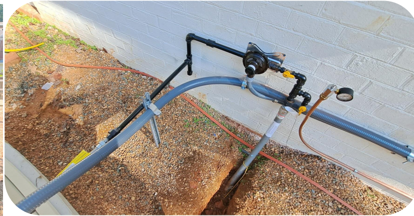
Phoenix Trimpe- AHS A generator he piped the gas line to.
